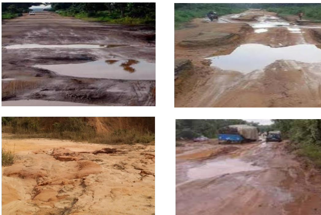
Figure 1: Some failed sections of the A123 Ilorin – Lokoja federal highway.
