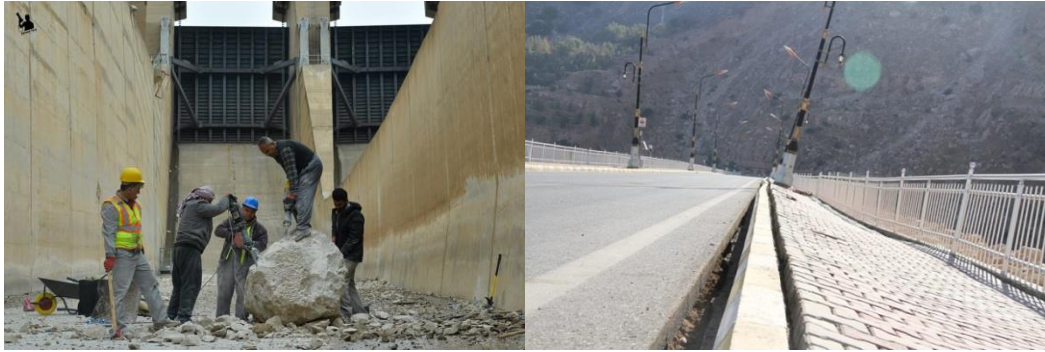
Figure 12: Aftermath of the earthquake in November 2017 at Darbandikhan Dam; a) Right: cracks in the main dam body b) left: group workers are demolishing a stone that fallen in spillway chute from the adjacent mountain.(Source:[18]).
