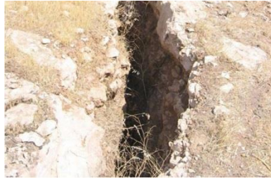
Figure 11: Upstream right abutment, open fissure resulting from slab sliding.
