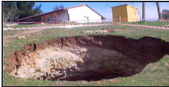
Figure 9: Left photo show the Ground settlement before the full development of the left bank sinkhole.
