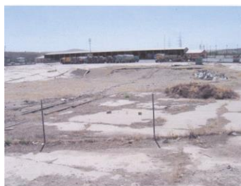
Figure 6: A sinkhole appeared during the 90's at the downstream right bank near the contractor yard.
