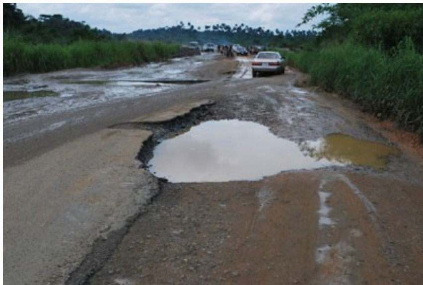
Figure 1: Typical pavement failure alongthe Calabar-Itu Road http://www.akwaibomnewsonline
