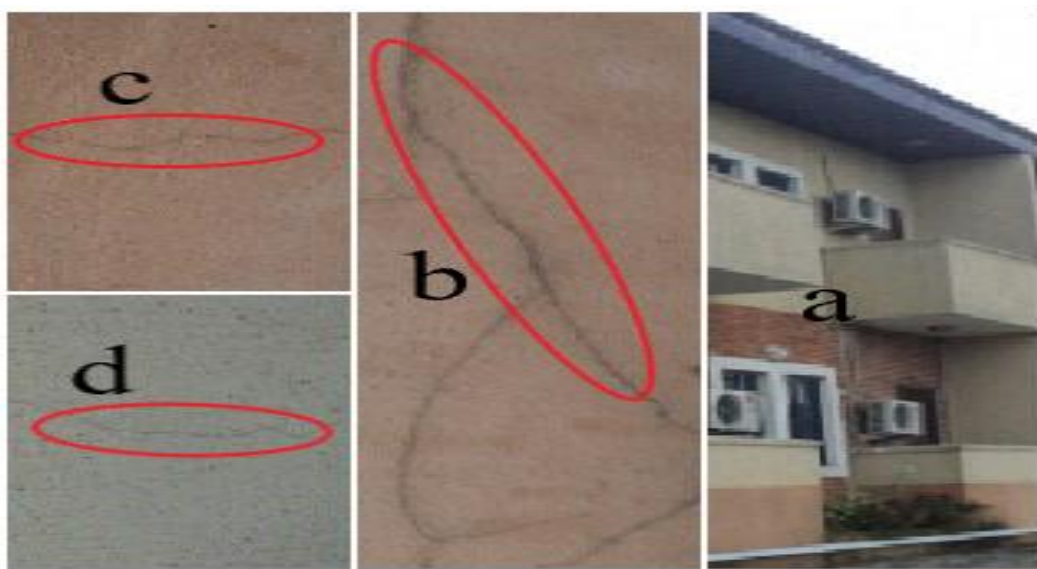
Figure 7: College of Technology Building, showing the severity of some diagonal and horizontal cracks on parts of the building (a) parts of the building under study (b) diagonal crack (c) and (d) horizontal cracks.
