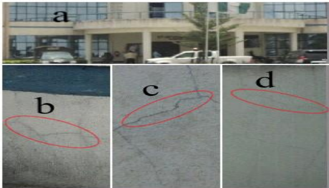
Figure 5: Administrative Building, showing the severity of some diagonal cracks on parts of the building (a) parts of the building under study (b), (c) and (d) some diagonal cracks.
