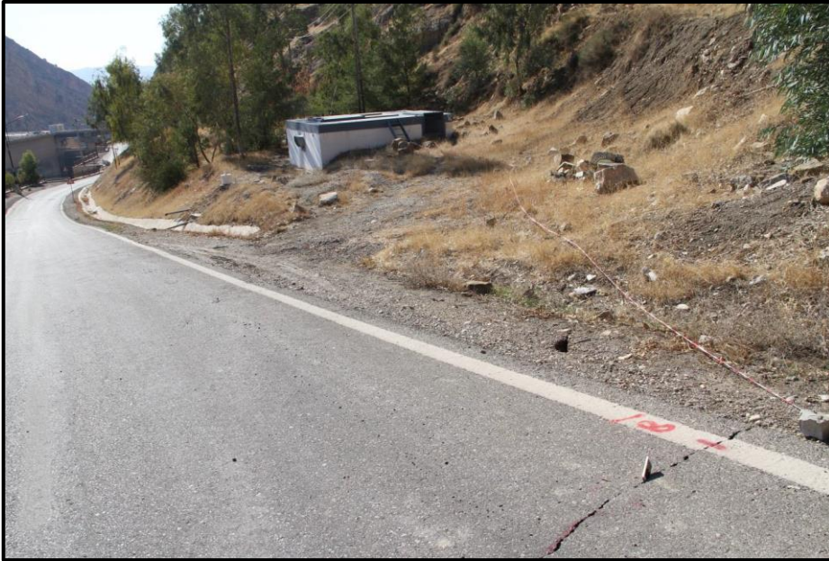
Figure 4: Location of a crack along the area above the landslide area (Crack is marked by red and white rope) and then extends down across the paved road down into the landslide area.
