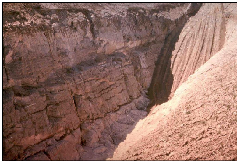
Figure 28: A view of the right abutment key trench showing the jointed nature of the foundation [34].
