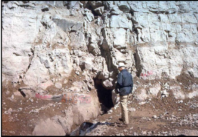
Figure 29: A view of a Large fissure in the right abutment key trench [34].
