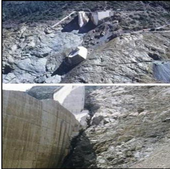
Figure 14-Top: the “dihedral” excavation with half of the thrust block fallen after the flow. Bottom: a wide crevice is open just upstream of the concrete arch, wider at the base and closing more higher [24].
