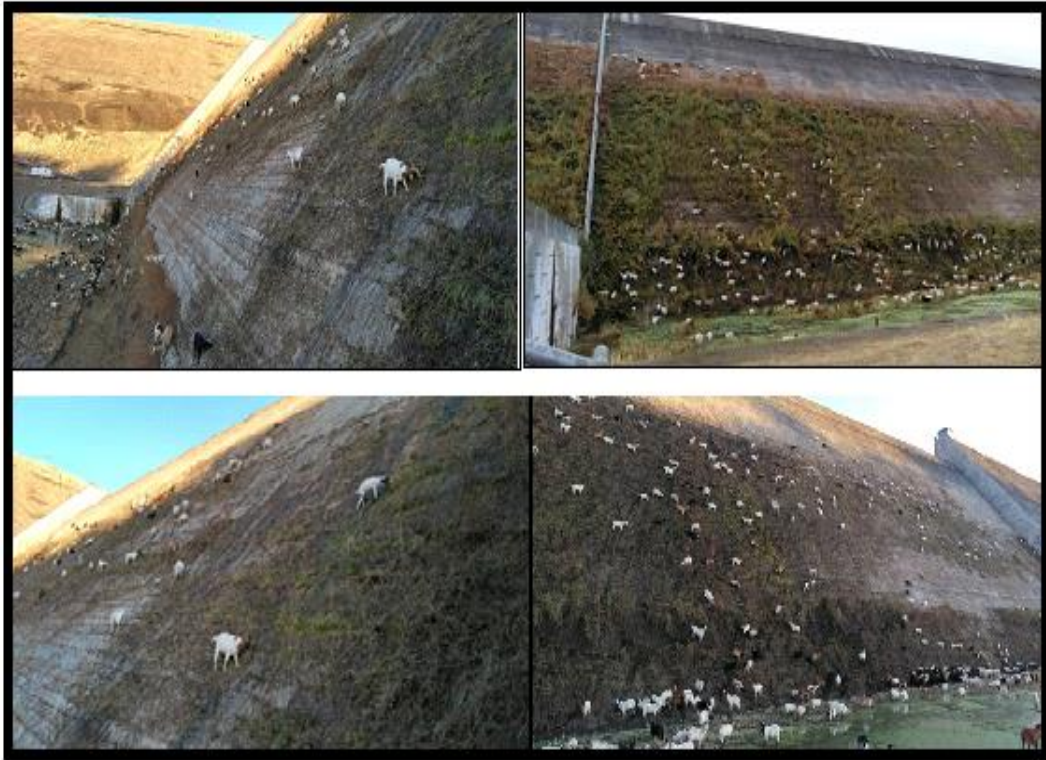
Figure 14: Leakage signs on the downstream side of the dam, and at the toe observe the heavy vegetation and the grazing goats [13].
