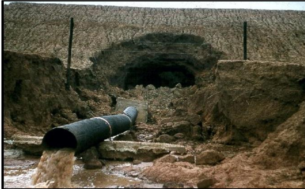
Figure 32: An embankment dam in Mississippi constructed of dispersive clay soil, failed on first filling with low reservoir level. Failure was likely caused by cracks from differential settlement, hydraulic fracture, or poor compaction about the outlet works conduit. The embankment dam had no filter and the clay was dispersive.
