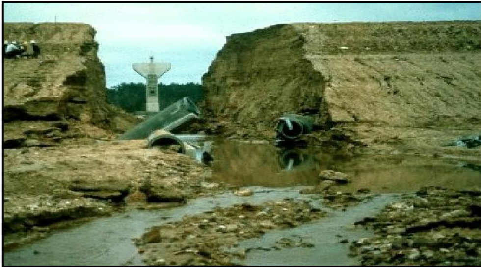
Figure 33: The embankment dam shown was constructed with dispersive clays, failed on first filling of the dam.
