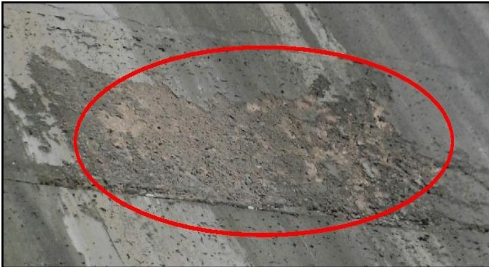
Figure 4: Disintegrating surface concrete observed on dam face.
