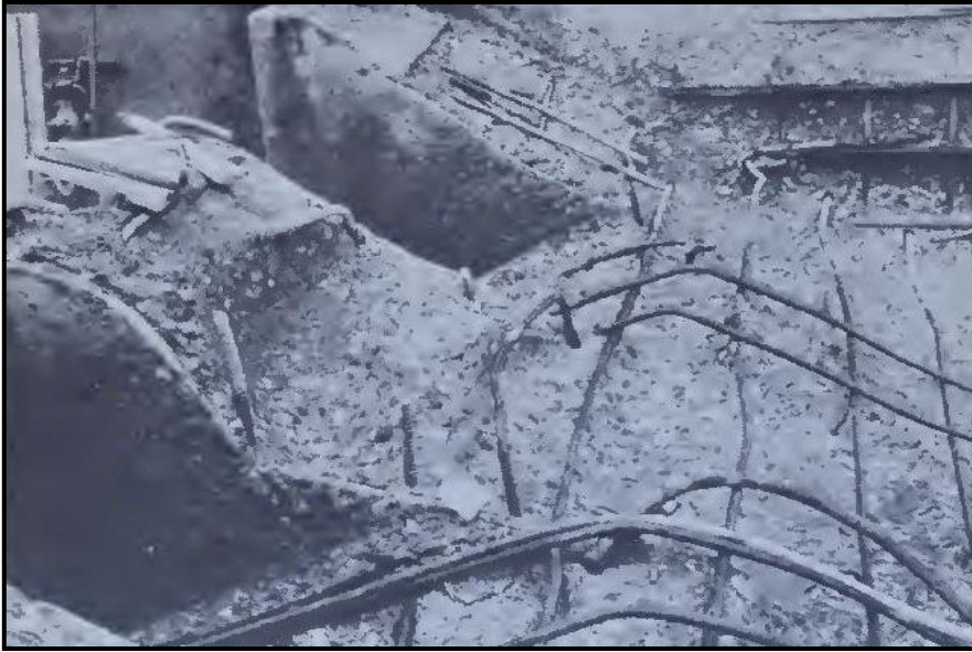
Figure 16: Abrasion erosion on concrete in the dentates, walls, and floors of the Yellotall Afterbay Dam Sluiceway stilling basin. The “ball mill” action of cobbles, gravels, and sand in turbulent water abraded the concrete, thus destroying the integrity of the structure.
