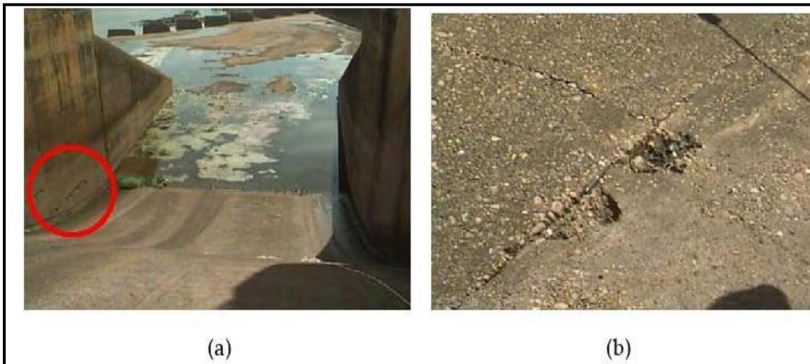
Figure19: (a) Dam Spillway deterioration by abrasion. (b) Defect in the concrete structure caused by abrasive process.
