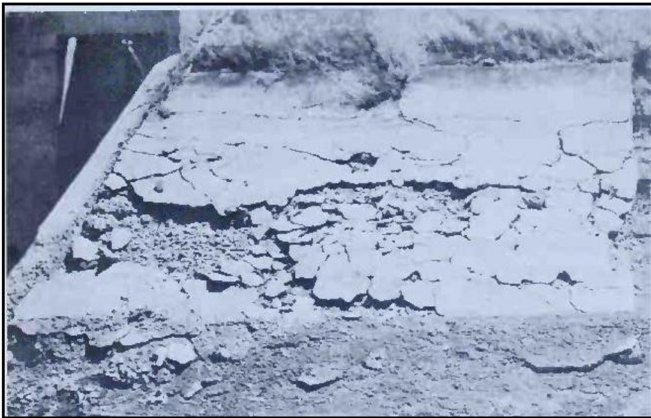
Figure 12: Disintegration of concrete caused by sulfate attack.
