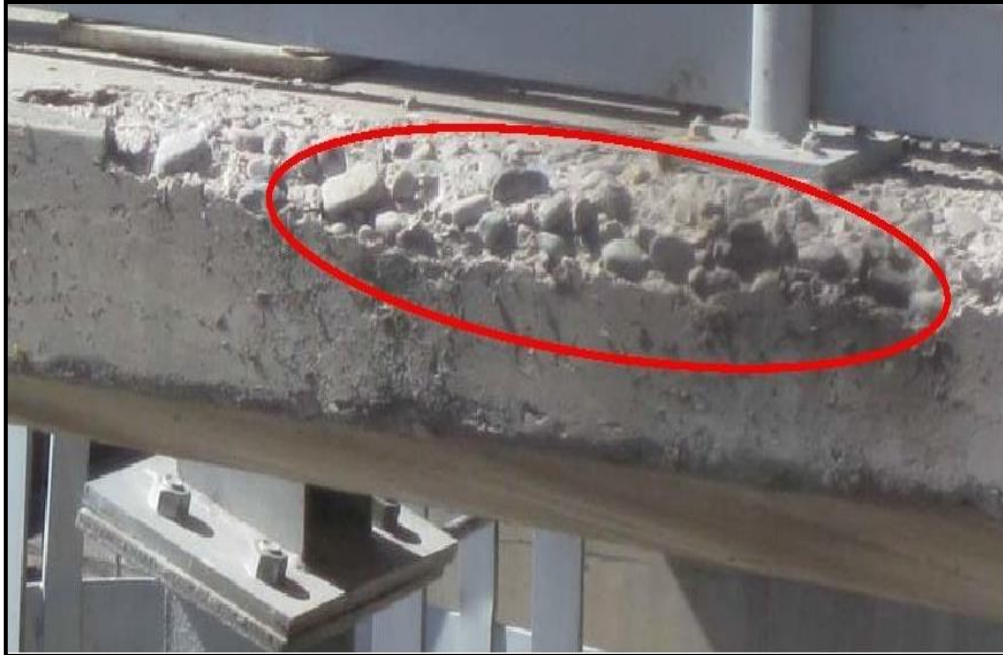
Figure 6: Structural deterioration of concrete on spillway gate operator deck. Extensive exposed aggregate is apparent.
