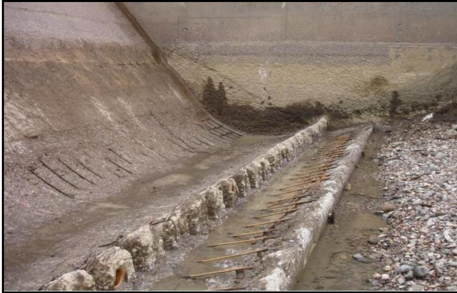
Figure 17: Abrasion erosion damage to the flip bucket and energy dissipators. The cause of the damage was not determined prior to starting repairs.
