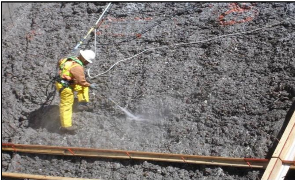
Figure 18: After beginning of concrete removal, the extent of damage became clear. Concrete was easily removed due to extensive deterioration.
