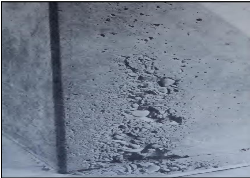
Figure 21: Cavitation erosion of concrete on a dentate in the Yellowtail Afterbay Dam spillway stilling basin. Fast-moving water during a flood flow, caused a pressure phenomenon at the concrete surface which triggered cavitation damage shown here.
