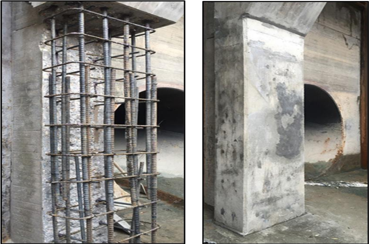
Figure 10: Repairs in river outlet works center pier showing reinforcing bars and the finished shape.
