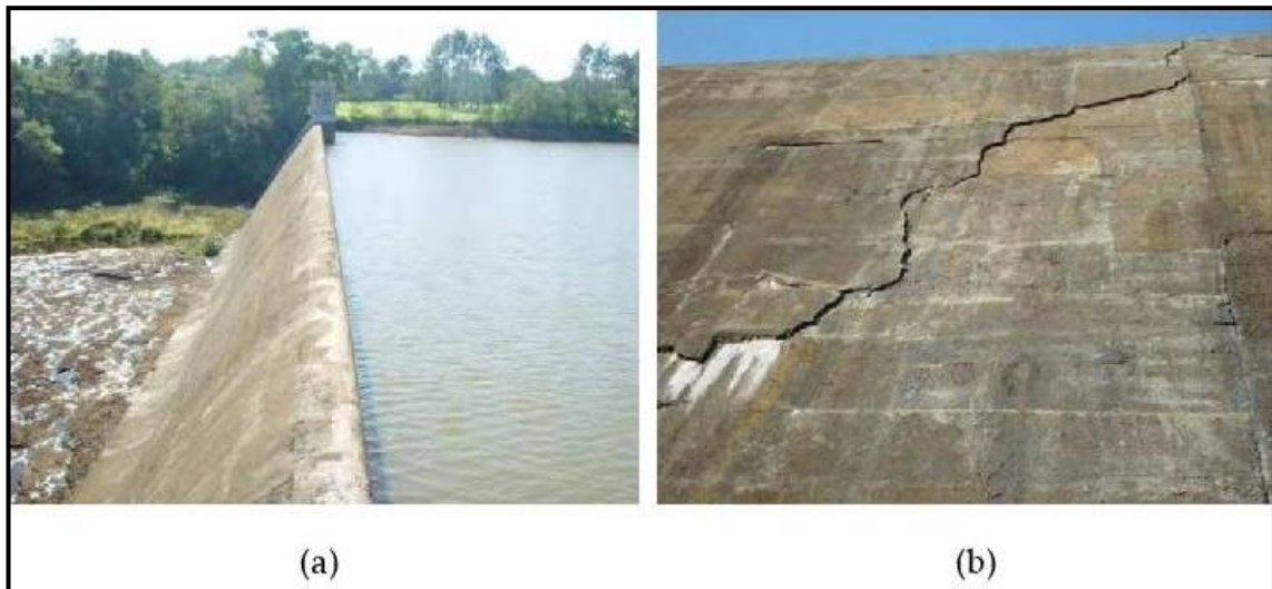
Figure 20: (a) Overview of the spillway of the dam. (b) Detail of the displacement of the surface caused by hydraulic abrasive processes.
