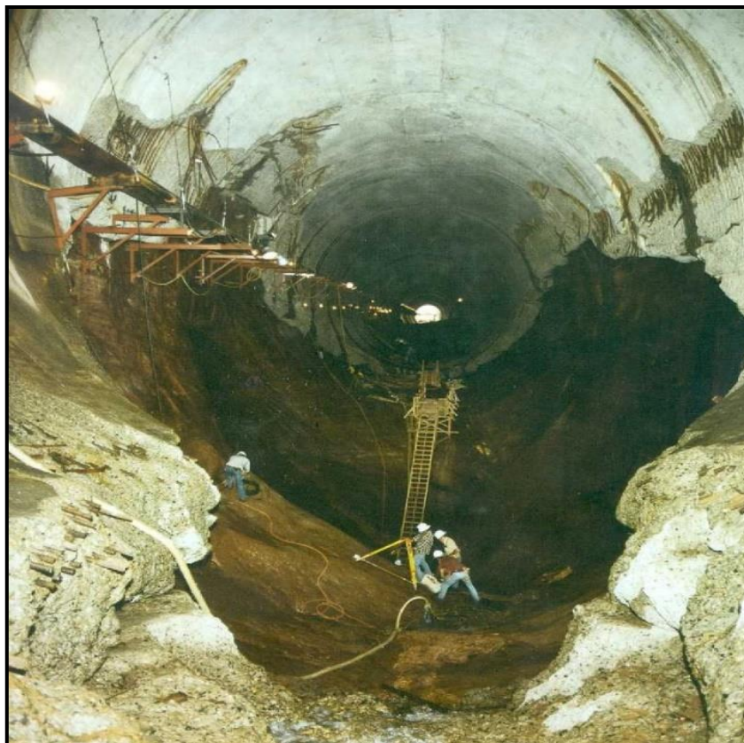
Figure 24: Glen Canyon Left Spillway Tunnel, September 1983. The "big hole" in the spillway invert was 11 meters deep.
