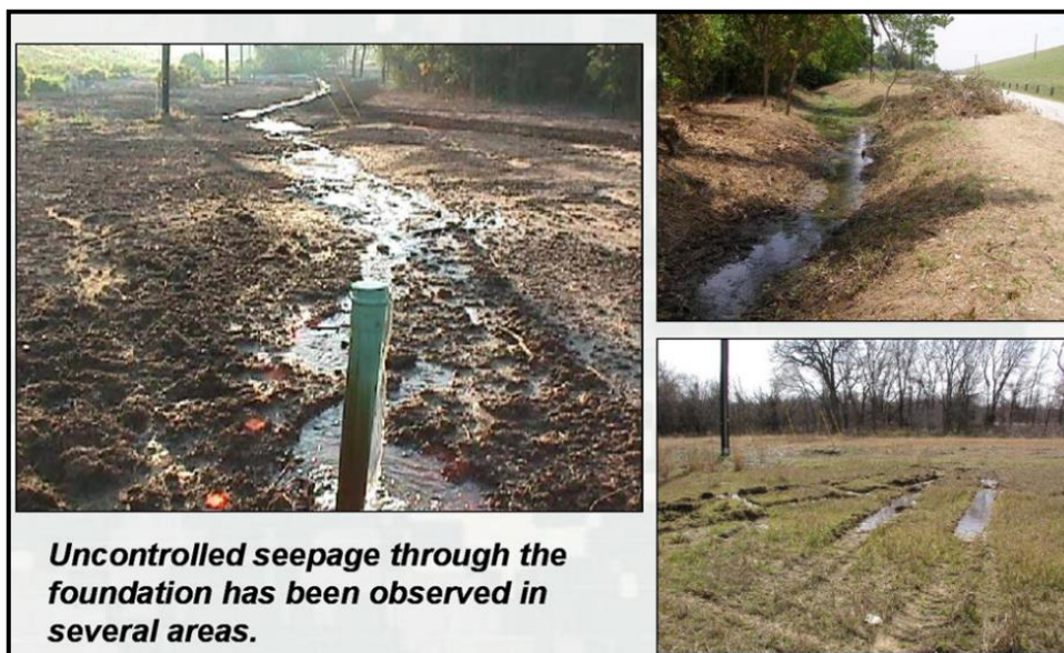
Figure 21: Uncontrolled seepage water from under the dam found in various area downstream.
