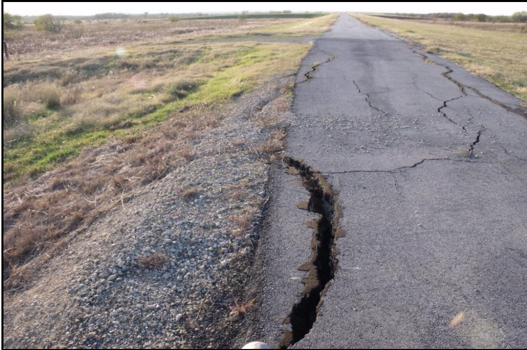
Figure 19: Typical cracking on Lewisville Lake Dam with clear signs of aging.
