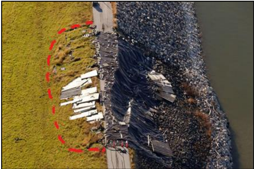
Figure 18: Slide area covered with plastic tarps, sandbags, and wooden planks for fear of heavy rain causing more damage [20].
