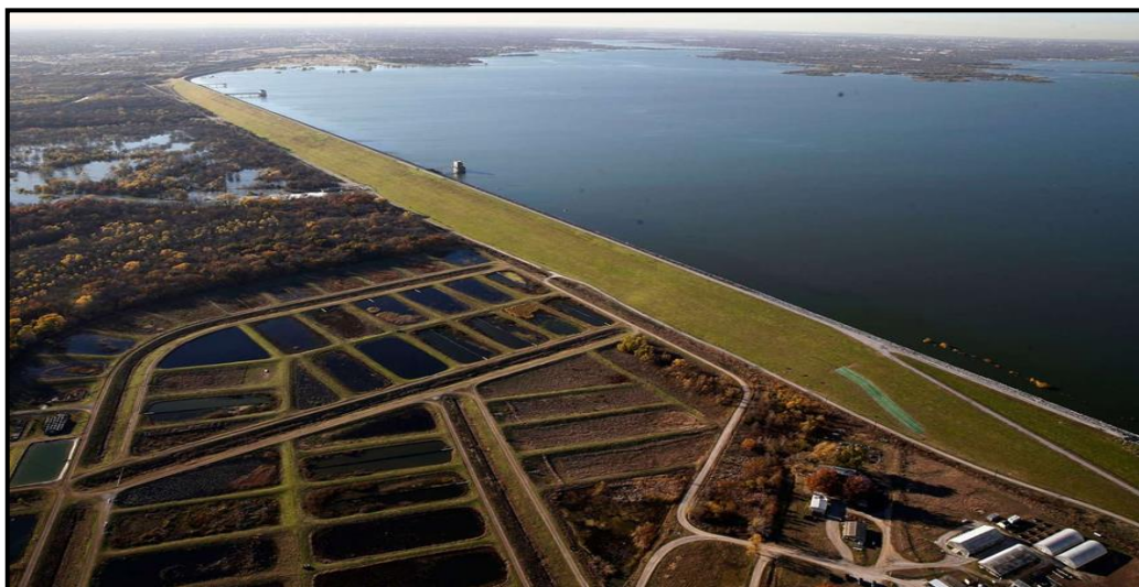
Figure 14: An aerial view of Lewisville Dam showing location of boggy area created by seepage.
