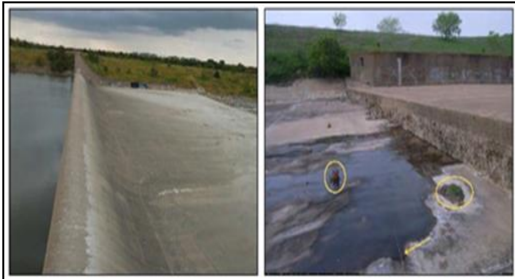
Figure 25: to the left, view of the Spillway when overflowing; to right view of the weir when not working showing cracks in the downstream apron.
