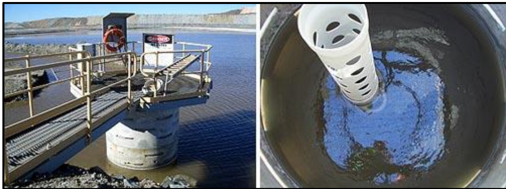
Figure 6: Decant tower with walkway (left), view inside the tower showing riser pipe and submerged decant collars (right) [15].
