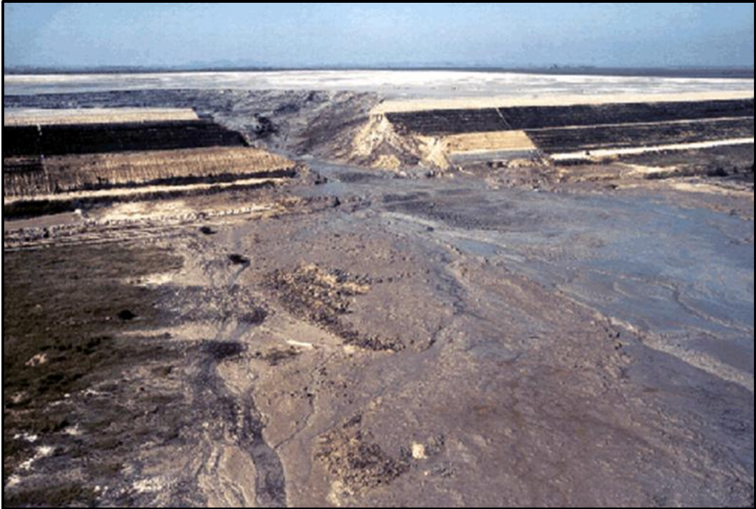
Figure 9: Close-up of the embankment breach.
