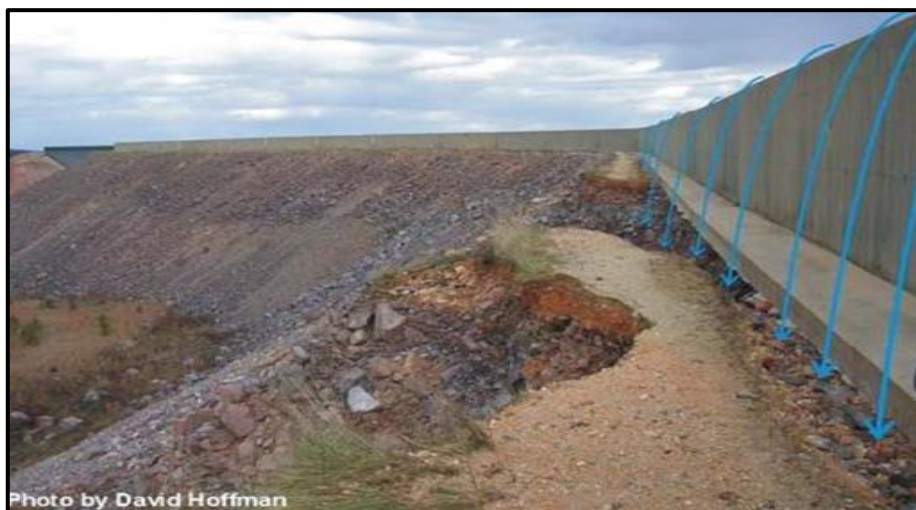
Figure 4: photo shows arrows representing the outflow nape once it extended beyond the wall footing and directly onto the underlying rockfill. The rate of scour and erosion increased dramatically once this occurred [3].
