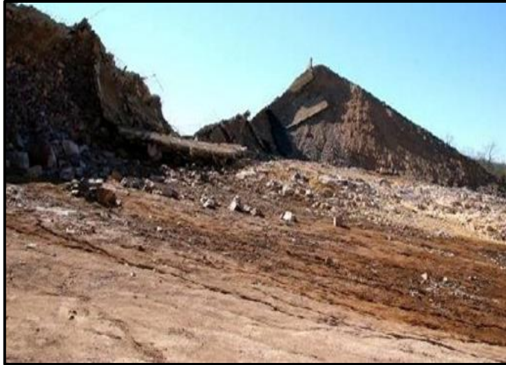
Figure 7: Photograph showing remnants of the lip as seen at the site of failure [3].
