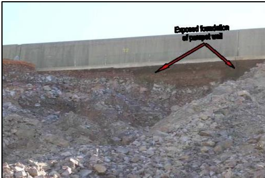
Figure 3: This photograph taken below panel 71-72 shows the deep plunge pool that developed and subsequently undercutting of the parapet wall [3].
