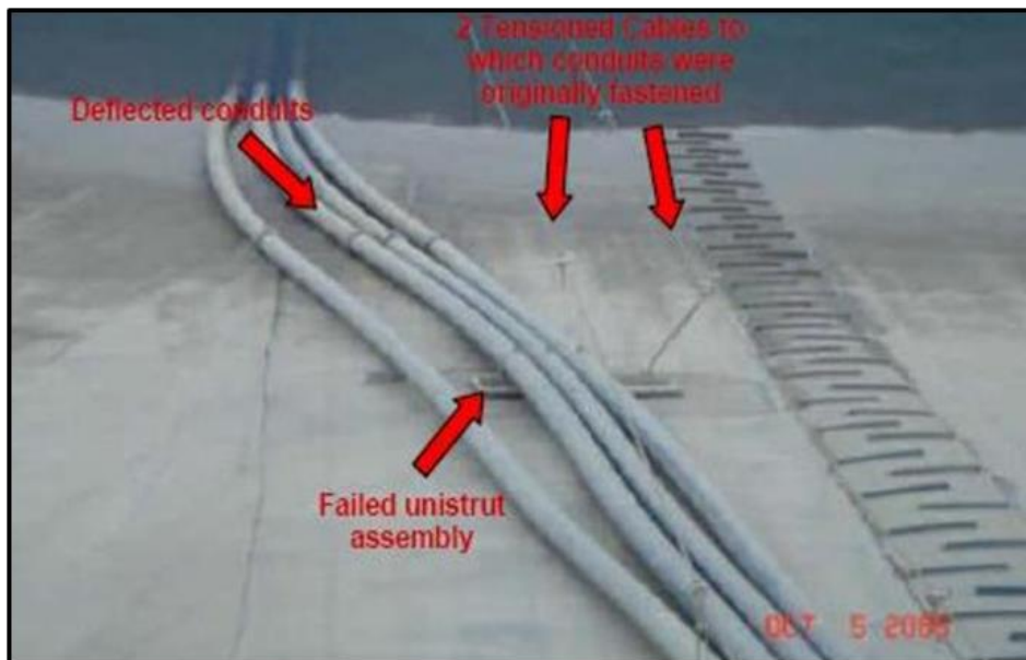
Figure 8: Deflected conduits at Taum Sauk Dam reservoir.
