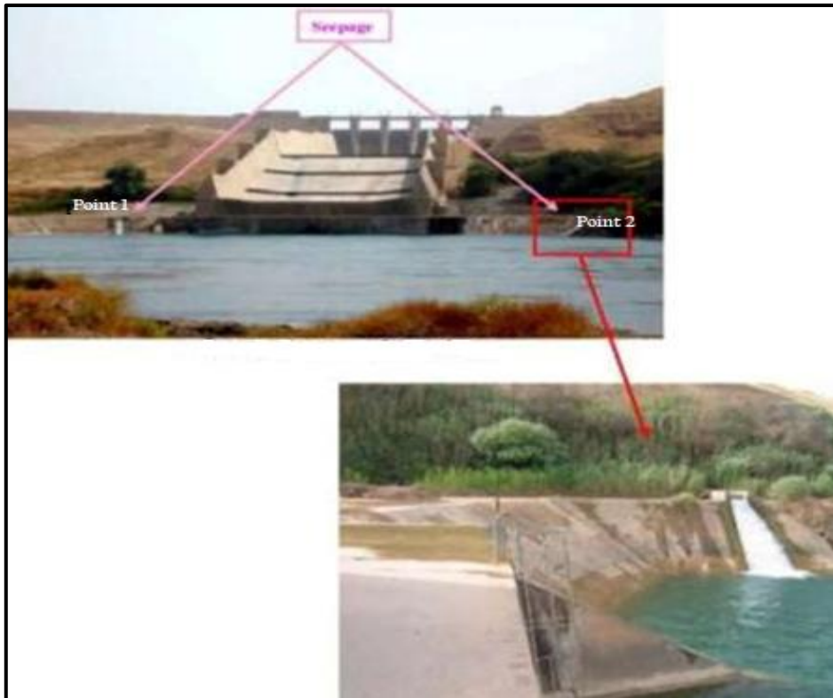
Figure 31: Seepage at left bank (courtesy USACE) [45].
