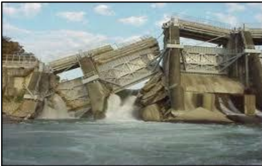
Figure 31: Shih Kang gravity dam immediately after the Chi-Chi Earthquake on September 21 st , 1999 [27].
