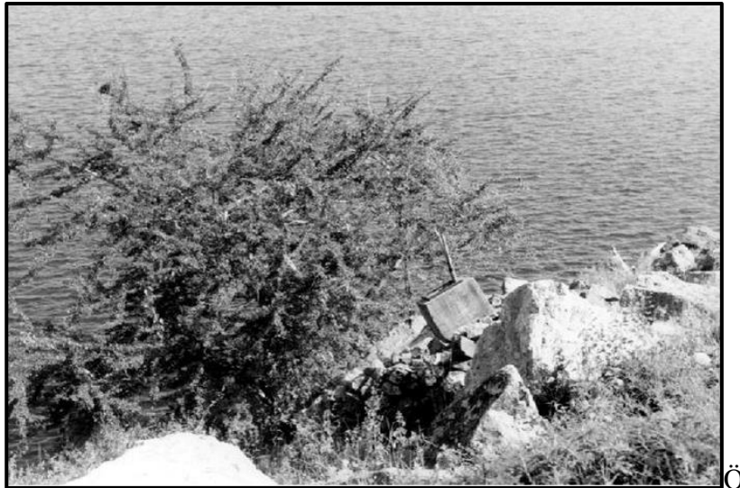
Figure 25: Settlement at piezometer box [22].
