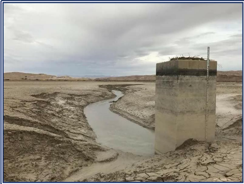
Figure 17: General view of Mandaly Dam Reservoir filled with sediments. (MoWR n.d.)
