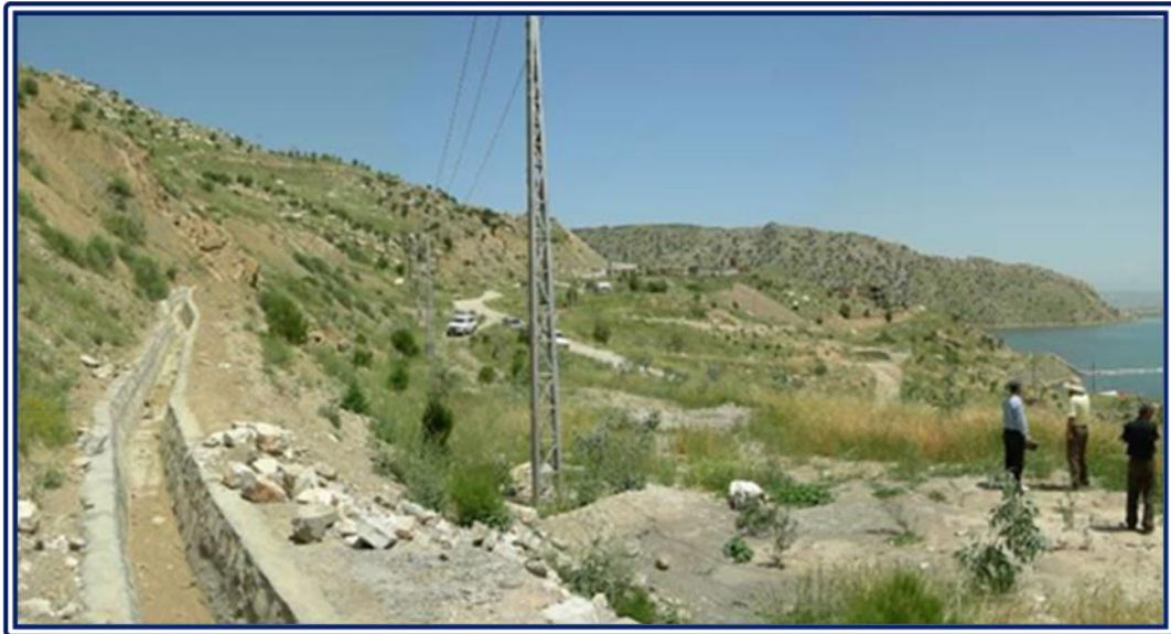
Figure 13: Land sliding on the right of Darbandikhan Lake (SMEC, 2006).
