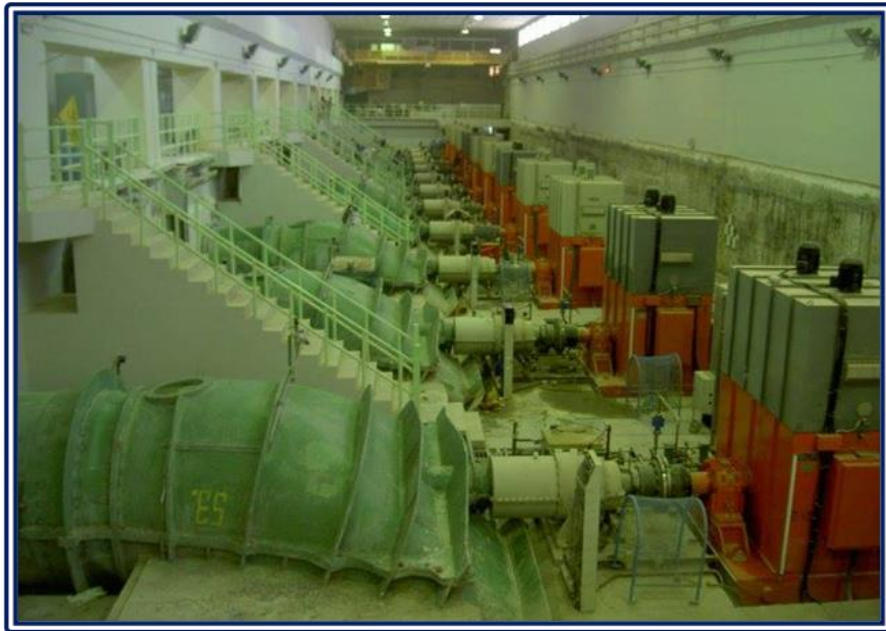
Figure 38: General view of MOD pumping station from the inside. (MoWR n.d.)
