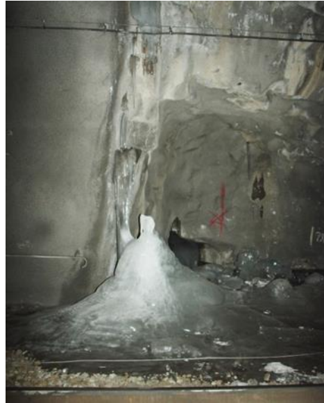
Figure 27: Ice pillar at the edge of the drain mat in the Glödsberget tunnel.
