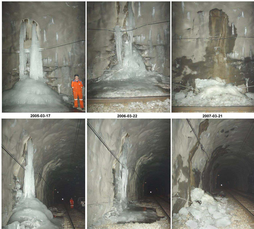
Figure 22: Comparison at chainage km 816+665 in the Glödborget tunnel in March 2005, 2006 and 2007 (Andrén, 2008).
