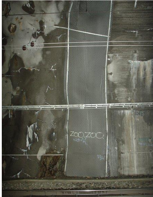
Figure 32: Uncovered drain, Kvedesta North chainage km 39+241 right, 2004-12-17 (Andrén, 2008).
