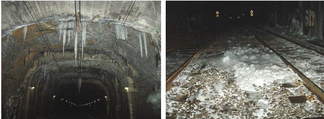
Figure 28: Icicles at an active leakage point and ice layers on the tracks, Rönninge South chainage km 29+720 the first picture photographed to the south, the second to the north, 2005-02-25 (Andrén, 2008).
