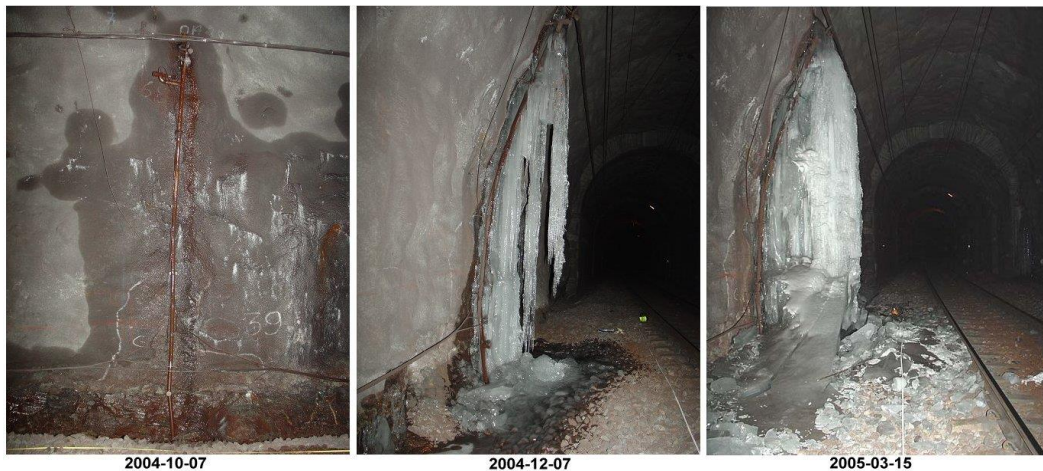
Figure 12: Drainage pipe, Nuolja chainage km 1512+610 left, at different inspections (Andrén, 2008).
