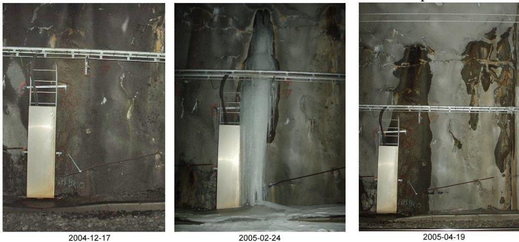
Figure 36: Differences between the three inspections, Kvestesta South chainage km 39+367 right (Andrén, 2008).
