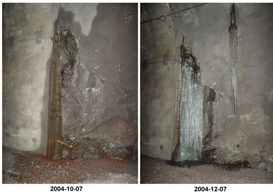
Figure 13: Water leakage where the rock and the concrete arches are connected. Nuolja chainage km 1512+626 (Andrén, 2008).
