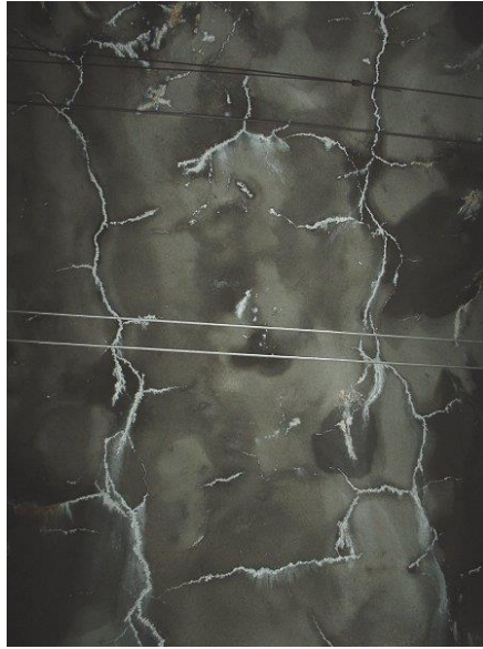
Figure 35: Cracks around a covered drain, Kvestesta South chainage km 39+372 left, 2004-12-17 (Andrén, 2008).
