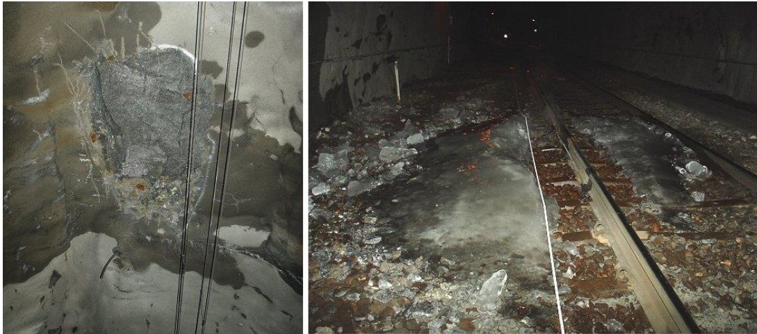
Figure 20: Exposed rock surface after scrapping of shotcrete and ice layer at the track, Glödborget tunnel chainage km 816+597, 2005-01-20 (Andrén, 2008).
