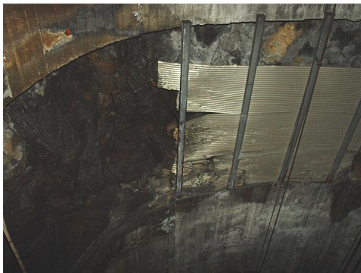
Figure 26: Sheet metal lying on beams between the concrete arches, Rönninge South chainage km 29+730, 2004-12-16 (Andrén, 2008).
