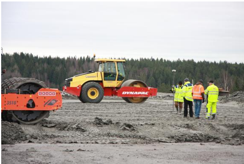
Figure 8: Smoothing of the upper surface for providing an even surface for the HDPE membrane.
